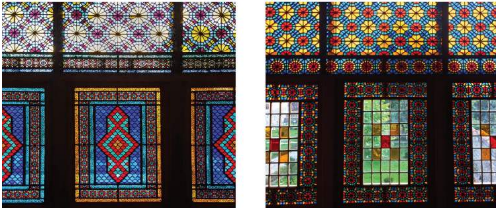
FIGURE 96: Restoration and conservation of decorative windows are carried out by local workshops engaged in the production of glass and wooden elements in accordance with the traditional typology.
