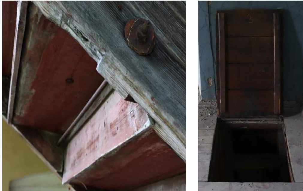
FIGURE 78: (a) The stringers are joined with metal rods fastened under the treads; (b) Access doors are installed at the end of the stairs leading from the ground floor to the first floor
