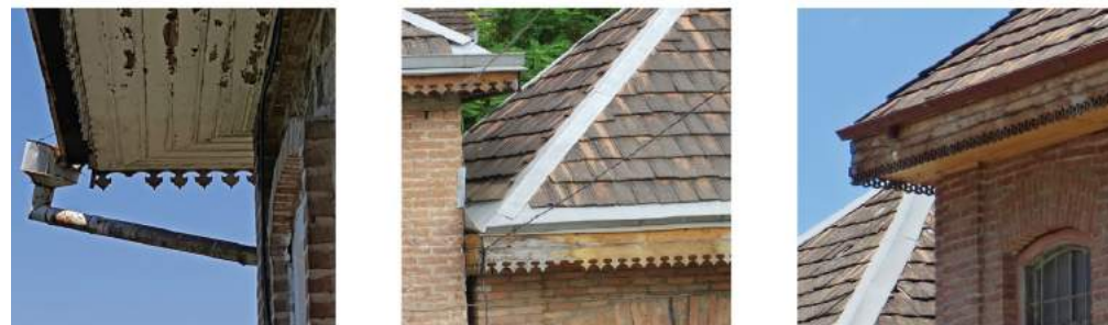
FIGURE 107: Wooden cornices are subject to rapid degradation with the detachment of sections. Wood loses its protective layer which should be renewed every five years.
