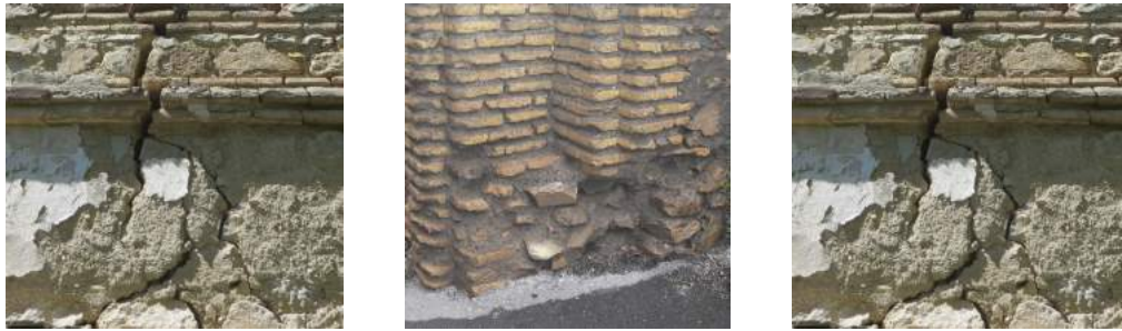
FIGURE 13: a) Influence of atmospheric factors on the lower part of the building; b) fractures caused by instability of foundations; c) reinforcement of foundations with concrete
