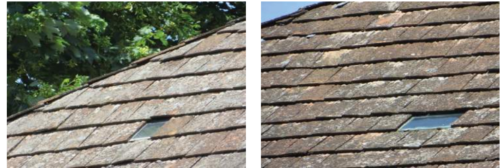
FIGURE 53: Simple skylights to allow sunlight into the attic making it habitable. The size of the skylight corresponds to one or two tiles.
