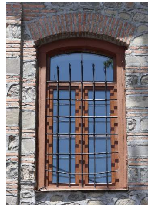
FIGURE 72: Correctly installed plastic window with wooden texture and wrought iron railings
