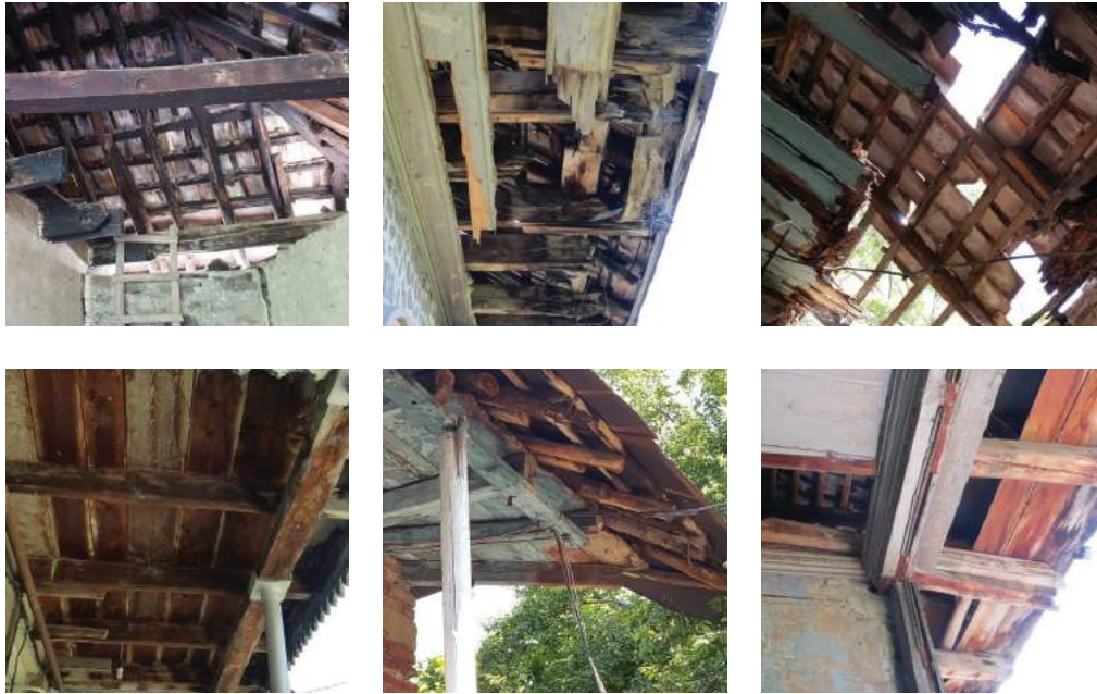
FIGURE 28: Moisture is one of the main causes of wood degradation. Causes of moisture include capillarity – the movement of water through the pores, hygroscopic effect – the absorption of moisture in the air, condensation of atmospheric humidity and infiltration factors.
