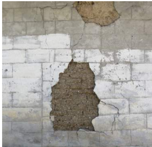
FIGURE 131: A plaster made of cement and sand on the wall made of mudbricks. Poor adhesion between two different kinds of materials, weak elasticity and airtightness of the cement resulted in the collapse of entire parts of the plaster
