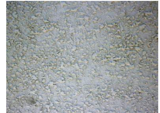
FIGURE 132: New types of plaster incompatible with traditional architecture include plastic-based sprays and rustic plasters made with sprayed mortar or cement techniques.
