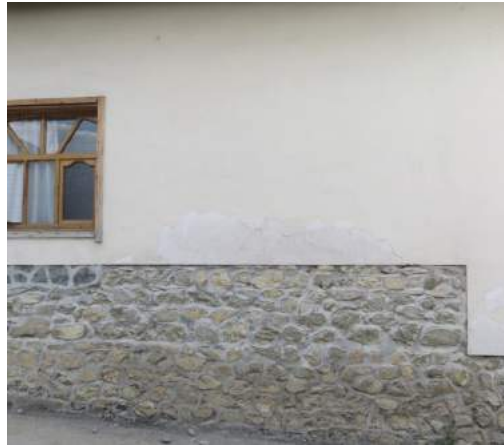
FIGURE 130: Traditional lime plaster is made in three layers, applied at intervals of time, to gradually cover the shrinkage cracks.
