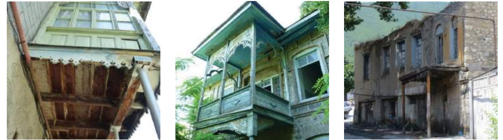
FIGURE 41: Decay factors for balconies and closed balconies are the same as the causes for degradation of wooden materials.
