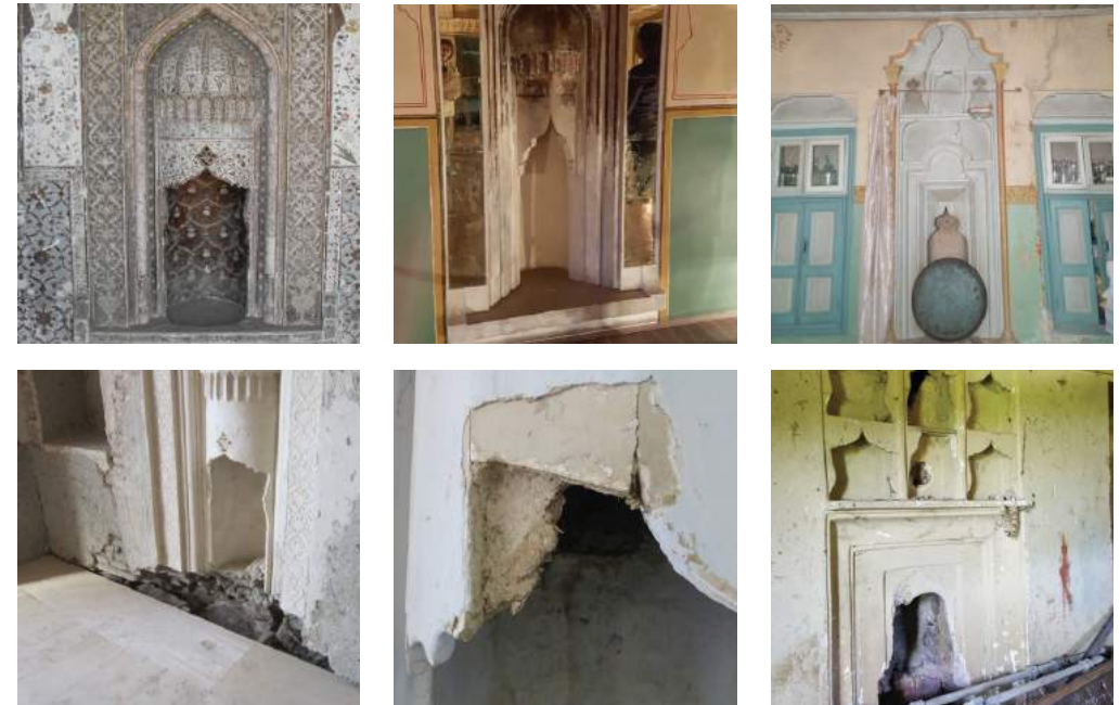
FIGURE 77: Most of the ancient fireplaces are currently in a dilapidated state due to being disused. They are subject to several factors of decay such as accumulation of alien elements, cracks, and loss of decorative elements.
