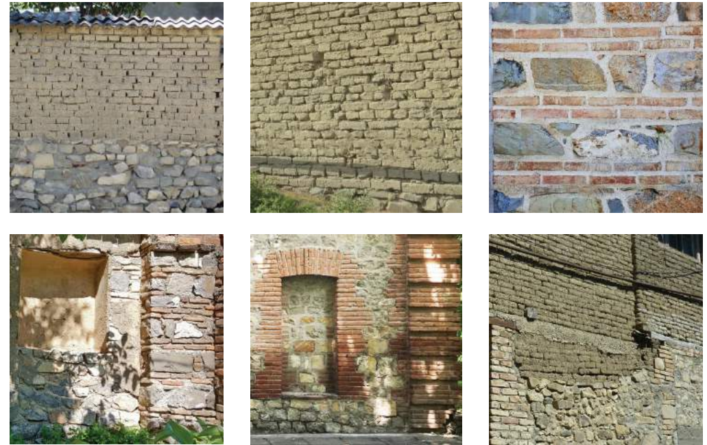
FIGURE 16: Mudbrick walls built in traditional style in the upper row; more modern masonry techniques of later periods using rock and fired bricks in the lower row.
