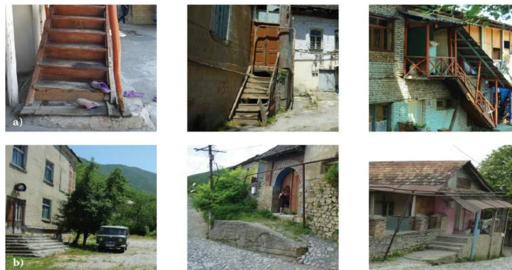
FIGURE 83: The causes for deterioration of stairs are the same as the causes for degradation of wood. Exposure to atmospheric elements, destructive activity of biological microorganisms, decay, etc. and the use of incongruous materials and forms that do not conform to traditional typologies.
