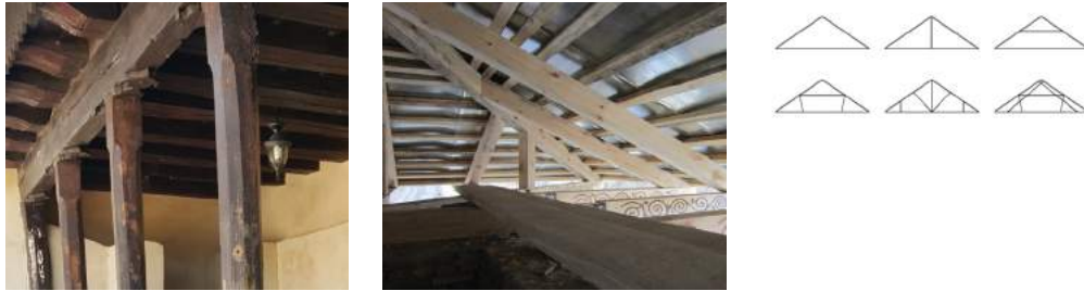
FIGURE 22: Attic structure in Sheki buildings are entirely or partially made of wooden joists, rafters, and tie beams.
