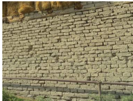
FIGURE 124: The most widely used material for buildings, since ancient times, is the rammed earth. One of its best uses is brick dried in the sun (adobe).
