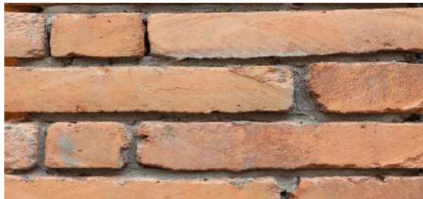
FIGURE 128: Brick cladding when only the façade of the building is covered with fired bricks.
