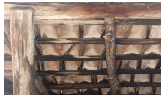
FIGURE 51: Wooden shims are placed between purlins and tiles along the joining lines of the tiles. Shims prevent any water leakage between two tiles. One of the most common cause of water leakage is loosening of shims.
