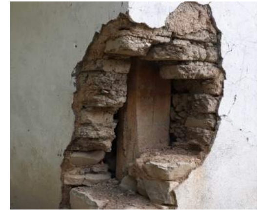
FIGURE 19: Wooden frame visible from the inside of the worn-out wall
