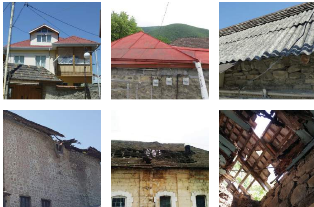
FIGURE 50: The main causes for deterioration of wooden structure of the roof are the same as the causes for degradation of wooden materials. Other causes include water leakage through gaps left by missing tiles, and contamination with modern roofing materials such as light grey aluminium sheets, asbestos-cement roofing or bright red modern industrial plates which come into conflict with traditional typology. Additions that are not typical of traditional roof shapes (protrusions, indentations, pocket terraces, etc.) should also be noted.
