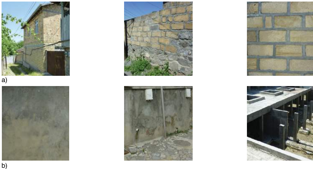
FIGURE 18: Modifications inconsistent with traditional materials and techniques such as (a) addition of lime-stones and (b) reinforced concrete structures with the help of cement-based plaster.
