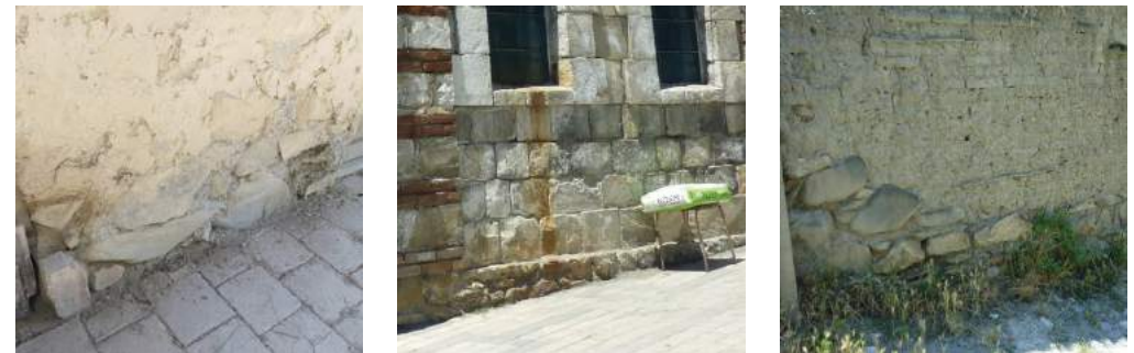
FIGURE 12: Stone foundations are laid from a depth of 60-80 cm to a height of 50 cm above ground level
