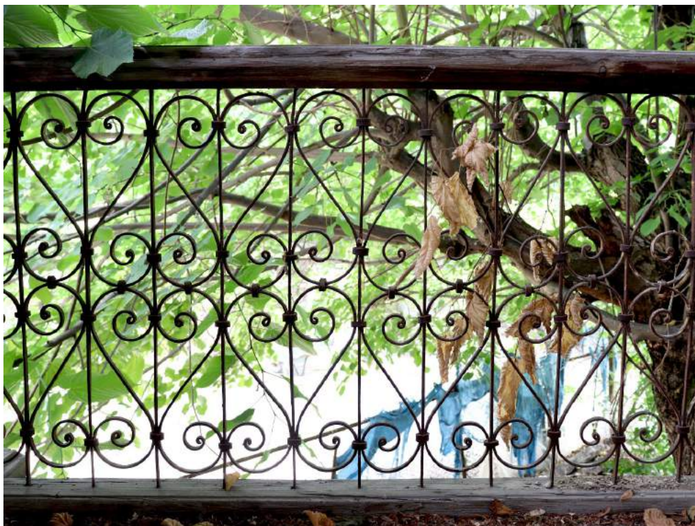
FIGURE 105: Balustrade made of forged metal
