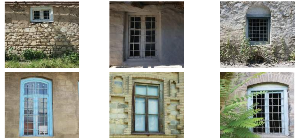
FIGURE 69: Traditional windows of Sheki are made of wood and have two or three casements. Windows on the ground floor have wrought iron railings outside.
