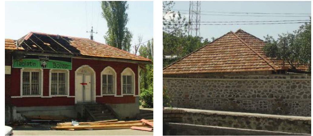
FIGURE 56: Various stages of the reconstruction of a traditional roof. The old roof, which could not be restored, is dismantled, new wooden structure is reassembled and then covered with ceramic tiles.
