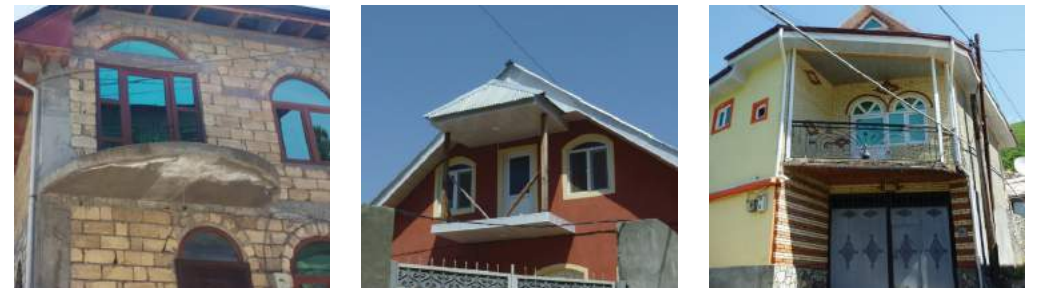
FIGURE 42: Another cause of decay of verandas, balconies and bay windows is complete replacement of existing elements or non-traditional architectural patterns in new buildings.
