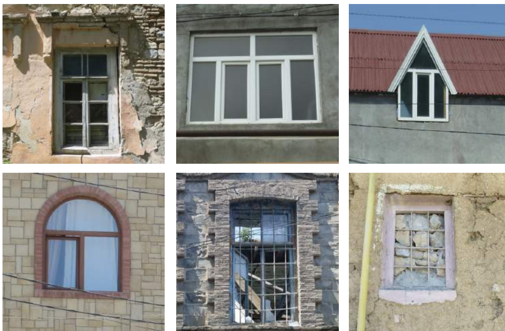
FIGURE 70: Some of the traditional windows in Sheki are in a state of decay. Wooden casings affected by xylophagous insects and atmospheric precipitation have deteriorated. Another factor of decay is the replacement of traditional wooden casings with modern casings that differ in both materials and forms.
