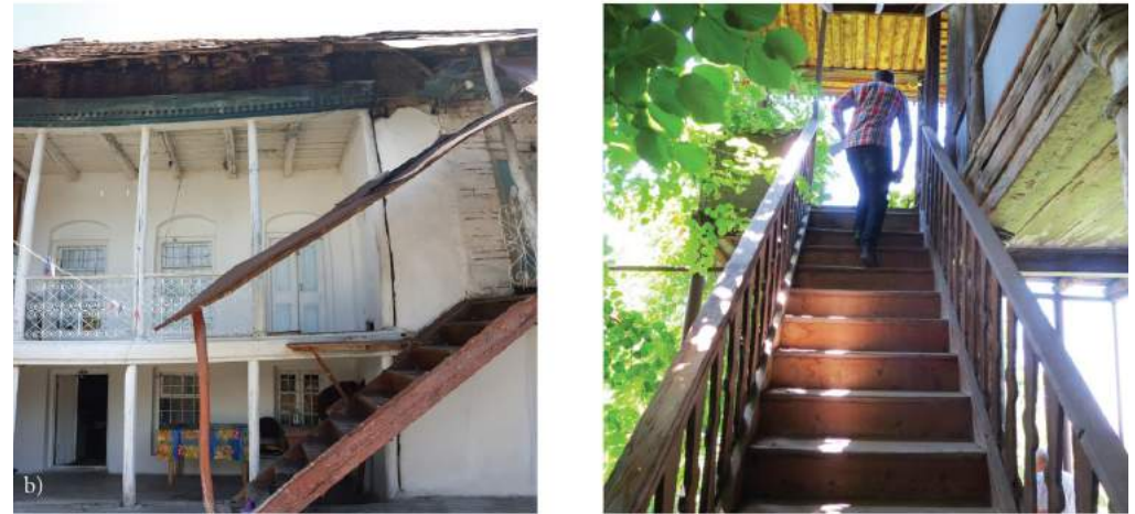
FIGURE 79: Typical stairs in Sheki only serve their primary function. They are usually in a straight run and made from masonry or wood.
